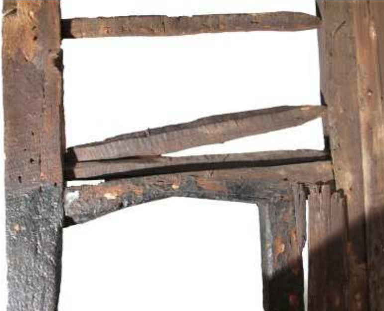
ground floor partition; false four-centred door head; staves for wattle and daub
