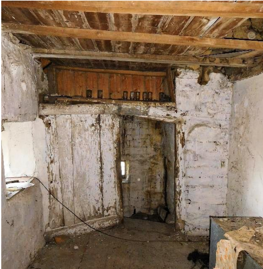
Above: Top of Llenyrch spiral staircase, with small window lighting it (Jenny Lees 2023)
