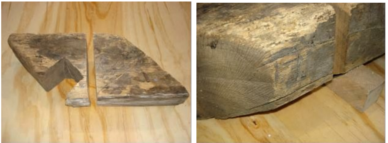
Fig 1a: Timber angg01 showing location of sample slice with II chiselled carpenters' mark
