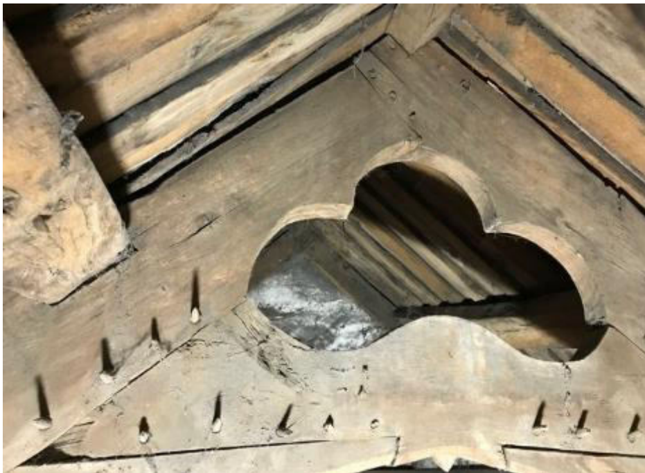
Truss now in Caenog attic with trefoil cusp and decorative pegs (Martin Cherry)
