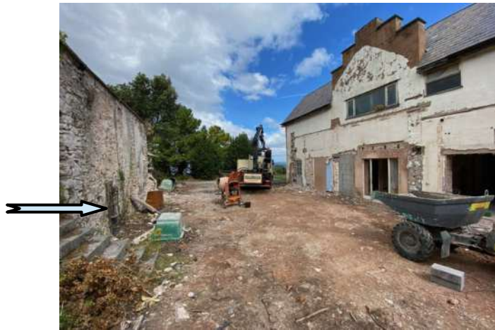
Pump and steps up into the upper courtyard. 2022
