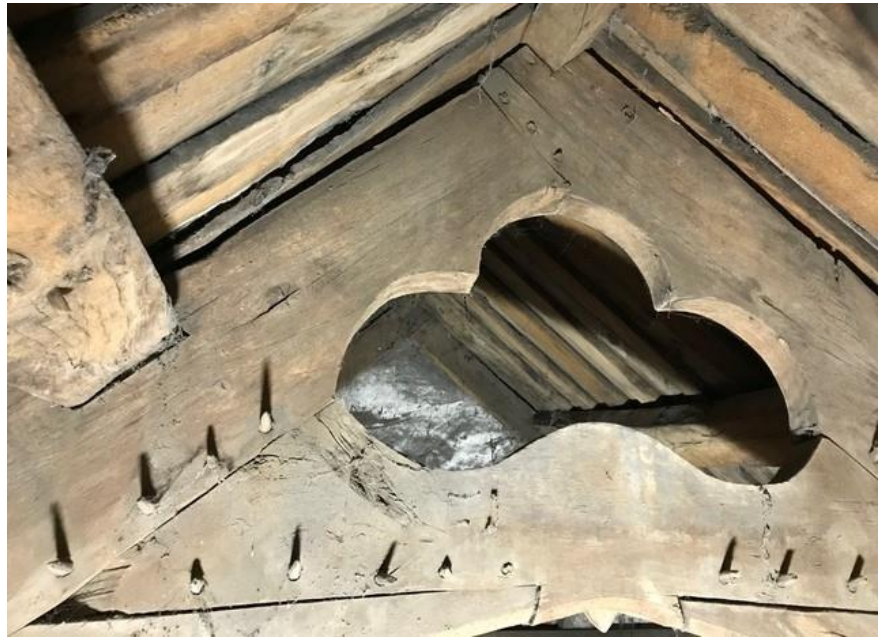
Caenog Roof over principal chamber with rebated boards between the rafters, a very rare feature Tree-ring dated to 1550
