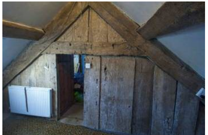
< ^ Typical burn marks beside door in loft screen at Llwyndu, Meirionnydd
