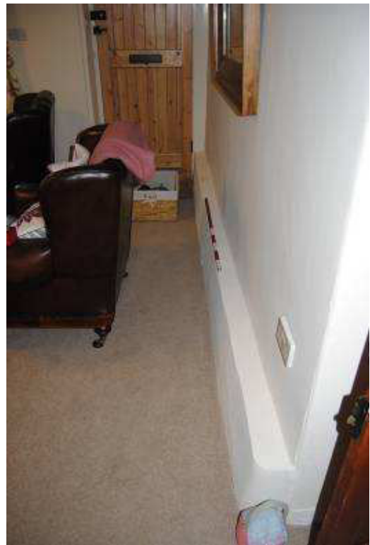
Plate 31: [GF03]; offset at base of east wall (ie. western exterior wall of primary range).
