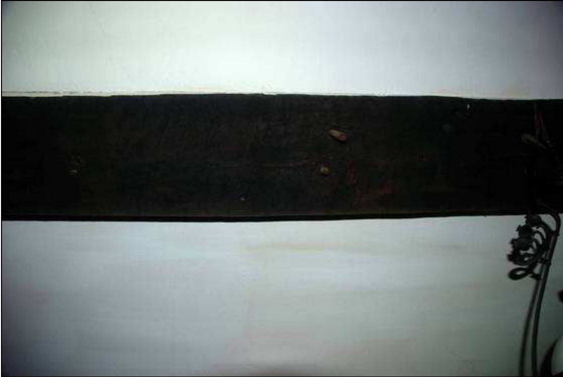
Plate 9: Pegs showing the positions of the common rafters attached to the lower front purlin
