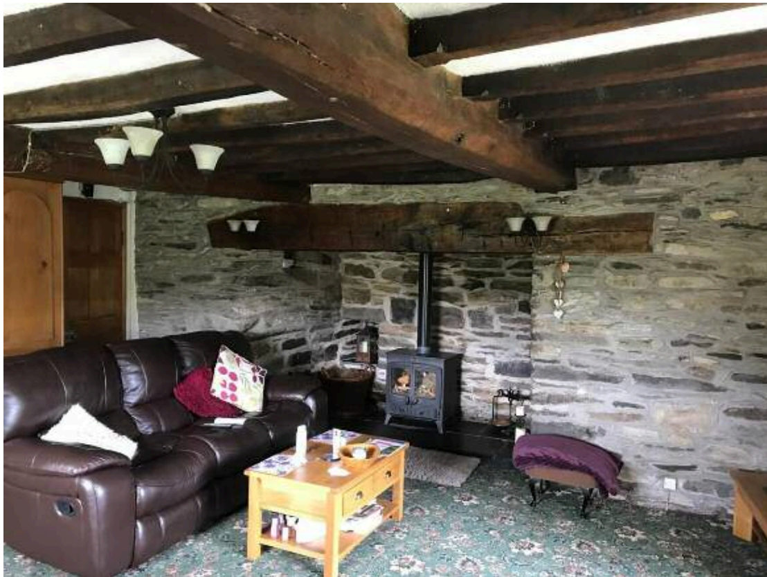
Fig. 4 – Parlour wing: ground-floor room, reconstructed after a fire, with slip tenoned joists. The chambers above this room were retained along with the principal rafter roof structure.
