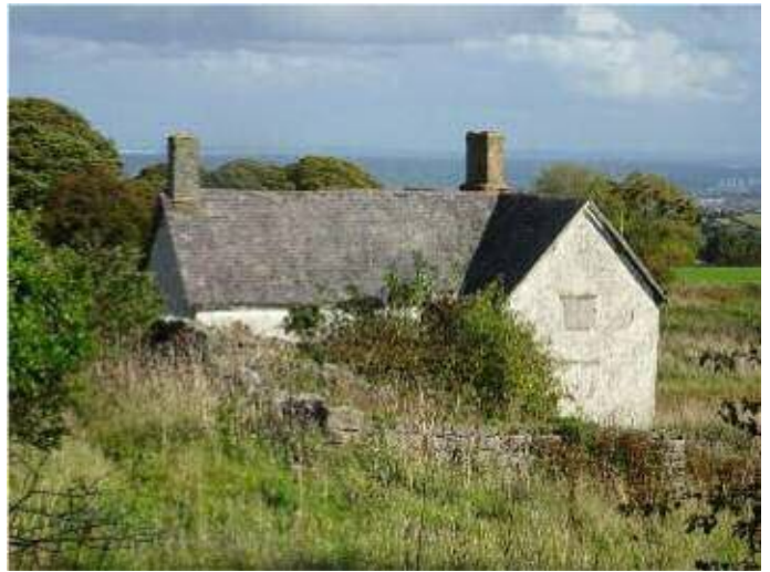
A historic farmhouse with a Jacobean staircase and a 1652 datestone in Brynford, Flintshire is on the at-risk register and is continuing to deteriorate. (Grade Two listed in 1962)
